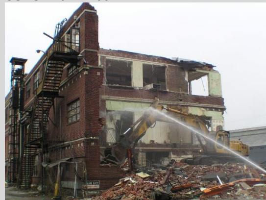
4.6 Sadly, one of the 877 photos taken during the 'demo' of the 'Main Office', which show great detail of the construction of the 'Main Office' Copy courtesy of SSHS 3 SSHS: h-041119021
