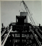
END OF LAST COLUMN SUBSTITUTED BY CONCRETE AS BE DONE WITH REINFORCING RODS ARE DETACHED IN PLACE ABOUT FOUR FEET OF SPACING UP END OF CONCRETE FORM. THERE ARE 44 FEET IN CONCRETE. ONLY REASON THEY STOPPED HERE WAS TO LEAVE WITH SPACING TO CONTACT WITH NEXT SET. (See photos, opposite.)
