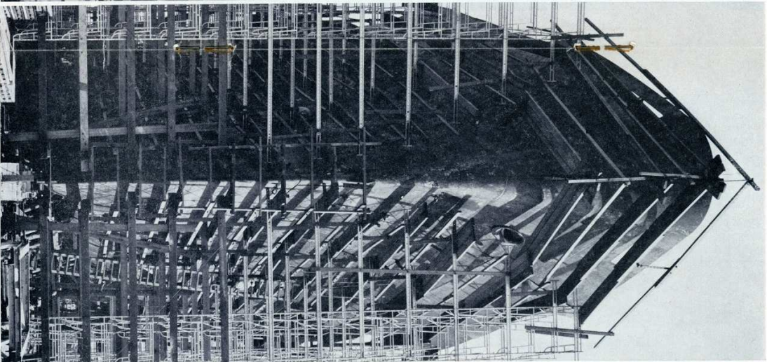
WE ARRIVE AT PLACE where no one now points in wonderment and says, "Is that a ship?" This is Hull #619 which is less than two months ahead of #620. Shell of hull is complete to the eye but much welding remains to be done and much of superstructure is unfinished. This vessel will be launched in about two months.
