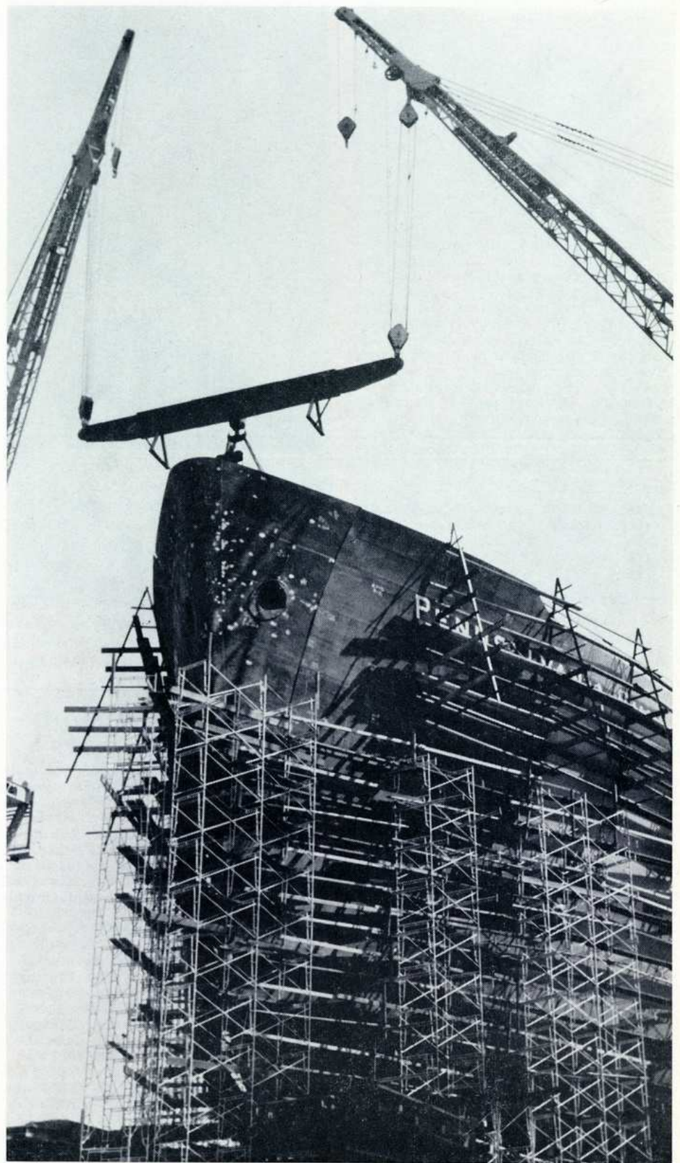
LAST OF THREE PIECES which formed bow section of Hull #610—pardon me, the Pennsylvania Sun—has just been set in place as gently as though it were a crate of eggs by two cranes at 6-Way. Of course this was like a basket full of chips compared to the other two 200-ton pieces (see the center spread in October OUR YARD if you have forgotten). For end result of all this effort see front cover.
