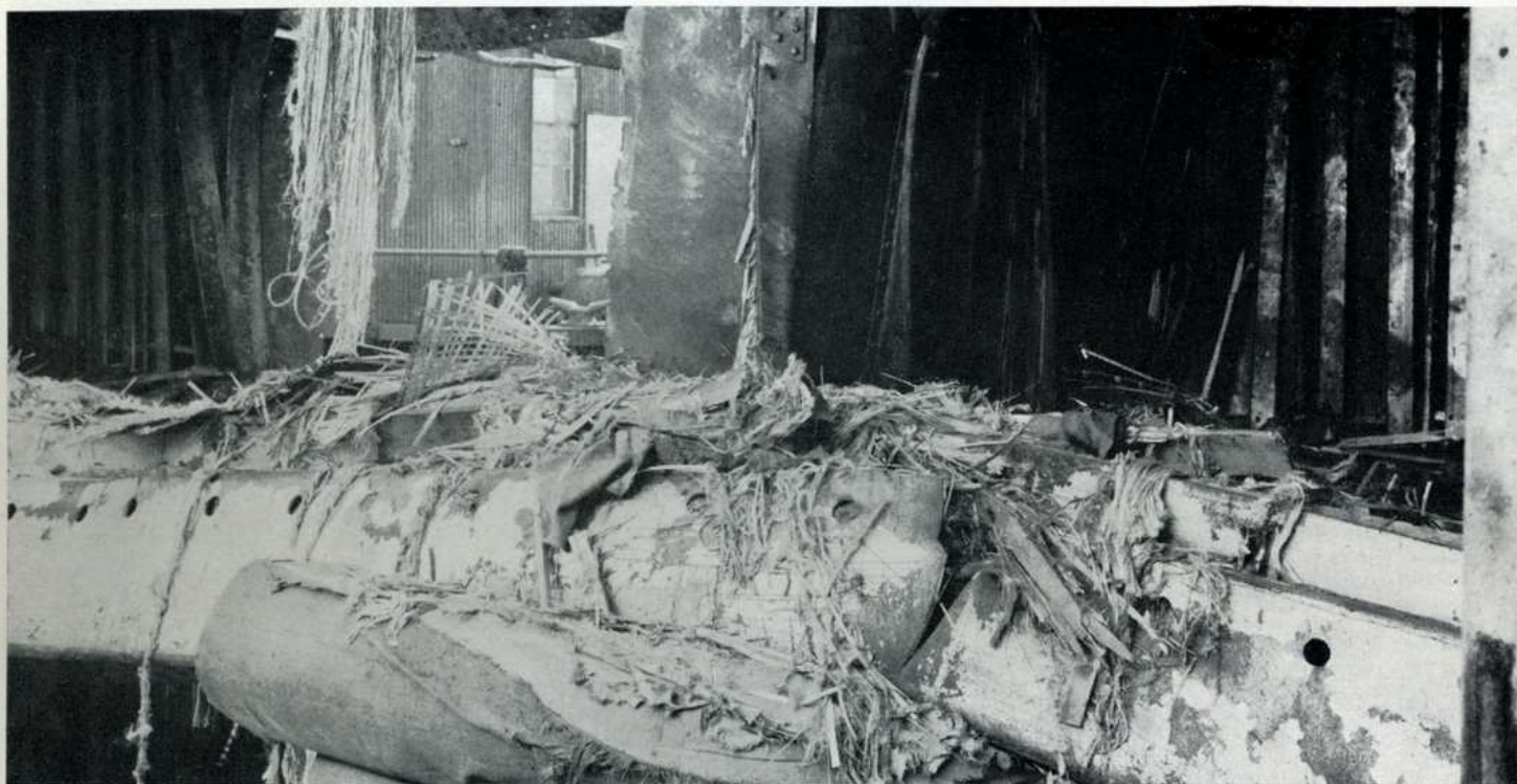
LOOKING OUT OF HOLD through gap in steel side of ship, dry dock office easily can be seen in background (above). Bundles (below) are lengths of 3-inch steel pipe wrapped in burlap. They were straight originally but were found bent to shape of tanker's prow after ships were separated.
