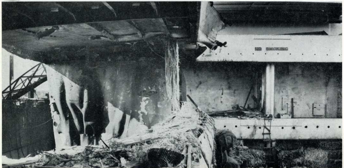
BOW OF TANKER was measured to fit. Rigger (above) stands on deck of Somerville over spot where tanker prow entered but steel beams supporting deck were sheared off (below) flush with underside of deck. Side of ship was rolled in like a curtain right down to keel plate. Hold largely was full of different materials to make rope (jute, hemp) which may have helped to cushion shock.
