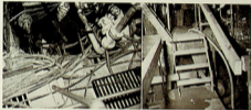
ENGINE ROOM STAIRWAY shows one step is floor and safe compared to similar location within another hull. Demonstrates why there is company rule forbidding the use of stairways and walkways for hose and cable, indifference or the worse!
