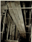
IMPROPER STAGING can lead to tragedy. At left, on, and pipe backroll is too far from the platform, no rigging, no safety netting. At right, a stagebuilder has balanced five short blocks on a pole suspended over a fire bucket, then tied a walking plank on top of the whole pile. (Note the timber extending into the hull which casts internal staging, hidden by sheetrock. If kicked away accidentally, an unsuspecting fellow angling the outside could have a terrible fall. The hands which built this monstrosity might have mused had the safety committee failed to see it, or not directed its dismantling.)
