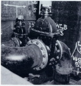
PIPE AND VALVE ASSEMBLY at bottom of a tankship's cargo tank, show: at top, the fittings which receive the shaft from hand wheels on deck forty feet above; and at bottom right, the bellmouth intake to the pipe system for pumping.
