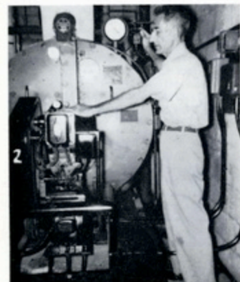
WESLEY HARDEN, formerly of 33 Dept., is presently employed as Chief Engineer in the Sorrento Hotel, Miami Beach, Florida. Here we see "Wes" checking one of the boilers which is one of his many functions. Mr. Harden and his wife, Sarah, reside in Northeast Miami.
