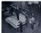
ON THE SHIPYARD DECK, some engine room construction within the ship's hull.
