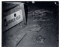
CONCRETE when installed was checked on floor to make sure the rollers on the belt track are correct. Each piece that fits in the conveyor top assembly is hand-fit to get into its track.
