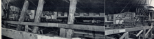
WORKER after and forward ends of the vessel, before the wedges are inserted to make the dging snug.
