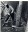
WORKER after and forward ends of the vessel, before the wedges are inserted to make the dging snug.
