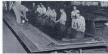
21—(LEFT) SECTION where template is placed on the steel for marking the fabricating pieces. Ledges (right, John Anderson, "Red" Tyndalick, Howard Hooley, Ed Pledge, Henry Kern, Ben Workman, Ed Peters and Henry Schickler.
