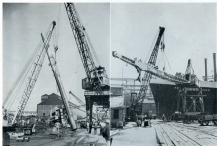
REPAIRS AND REERT shows workers setting new beam in place on Shanty crane. ON SHIP is a view of the barge that moved cranes after its load beam lifted from the water. Shanty cranes are able to move loads in water.
